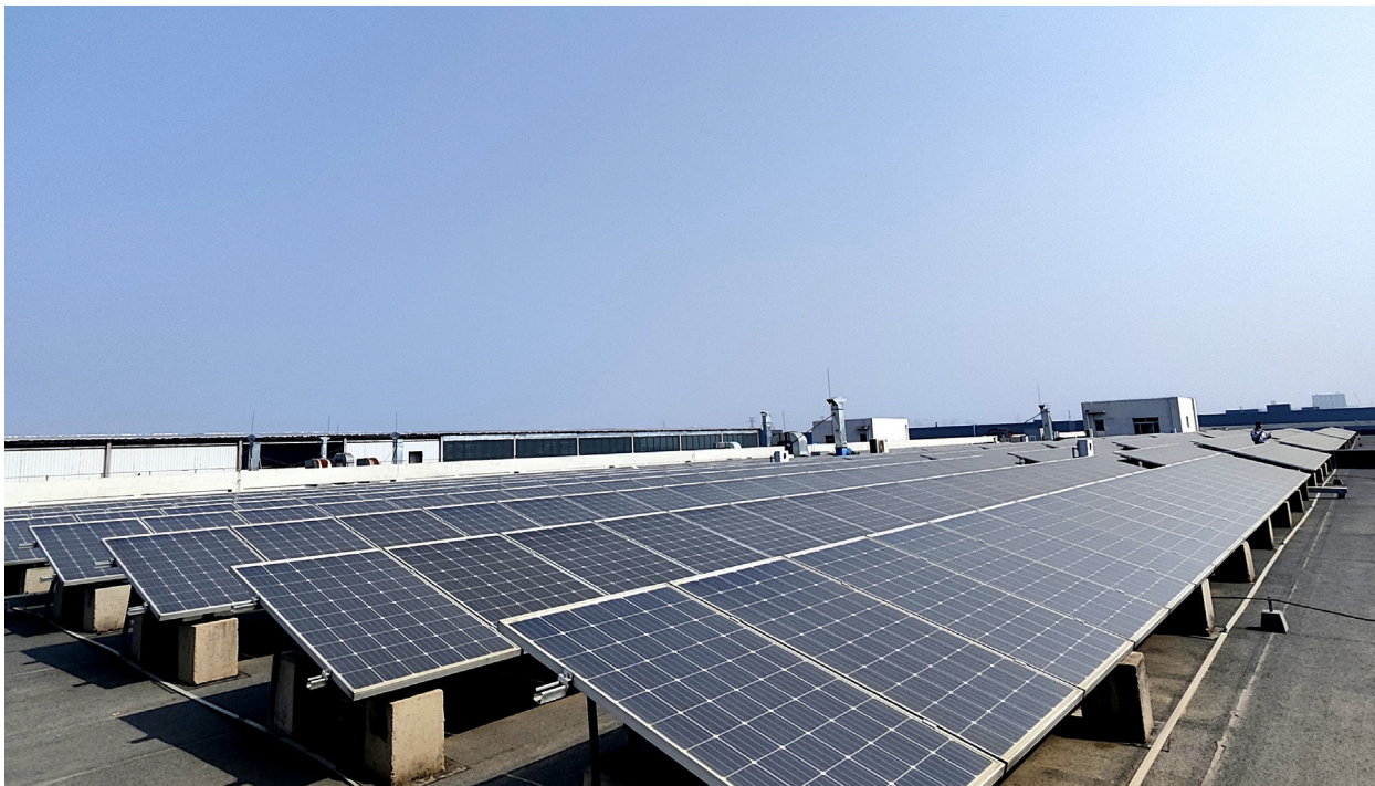
Rooftop PV plant in a supplier's factory
